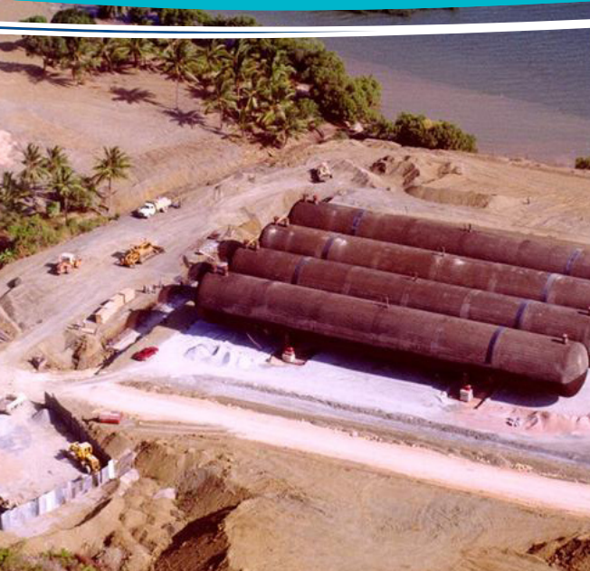
LP Gas import facility Mombasa, Kenya
